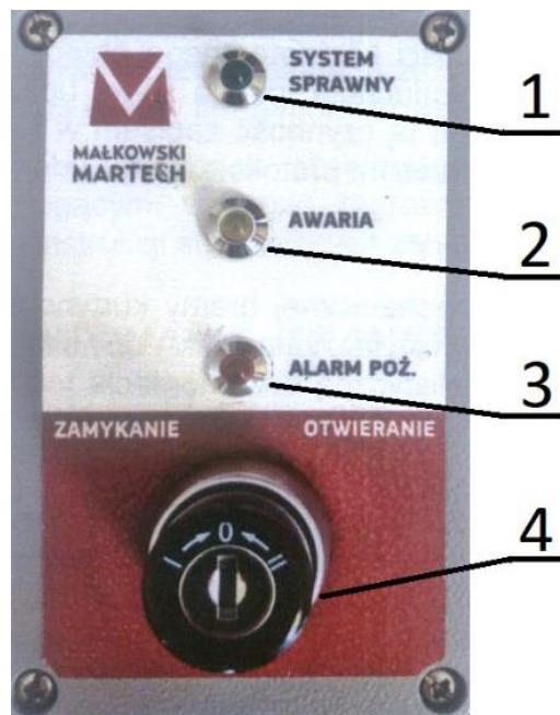
Figure 1. Key-operated switch for fire protection curtain gate.
